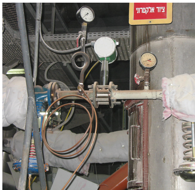
An inline wafer multivariable steam meter is used to measure and control steam at an animal food plant in Israel. The steam is injected into the dry pellets to give them constancy and uniformity.
